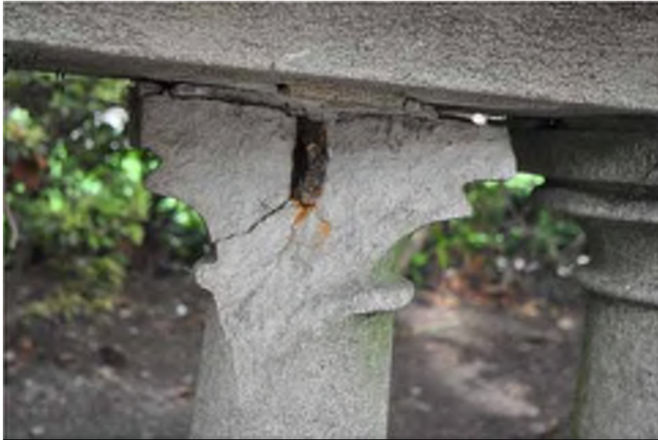
Figure 1: Spalled stone due to rust jacking at a railing. Credit: Brian Rich, 2013
