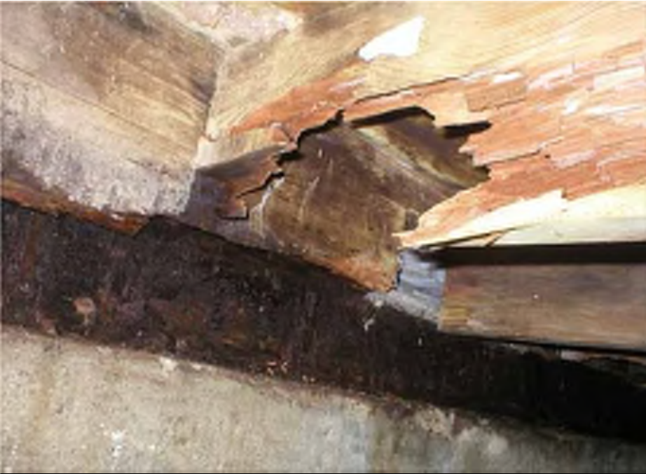
Figure 5: Rotted wood due to improperly installed membrane or siding. Credit: http://www.moldknowledge.com/dry%20rot%20photo%206.JPG
