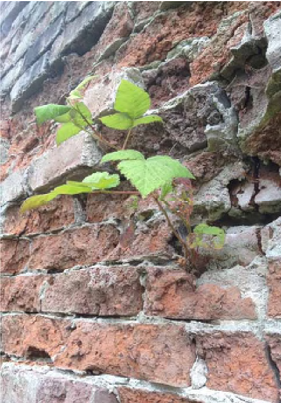
Figure 0: Brick and mortar deterioration at an exterior site wall. Credit: Brian Rich, 2013
