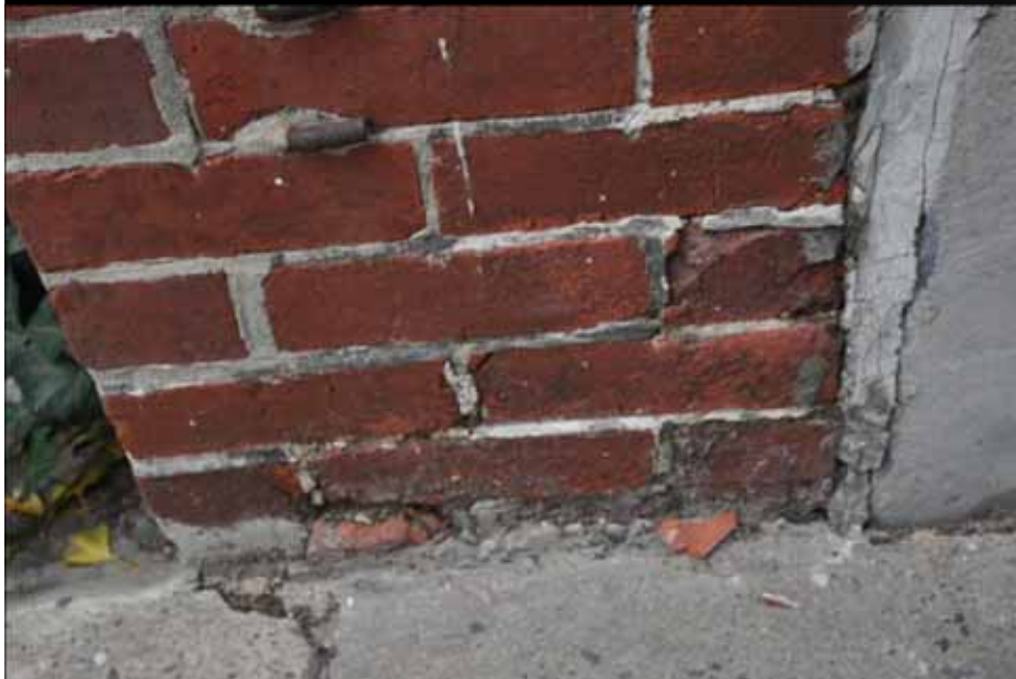
Figure 2: Brick spalling due to mortar installed that was harder than the brick. Credit: Brian Rich, 2013
