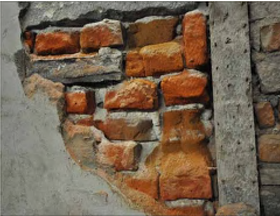
Figure 3: Deteriorating brick, mortar and plaster at the barracks at La Citadelle de Quebec. Credit: Brian Rich, 2014
