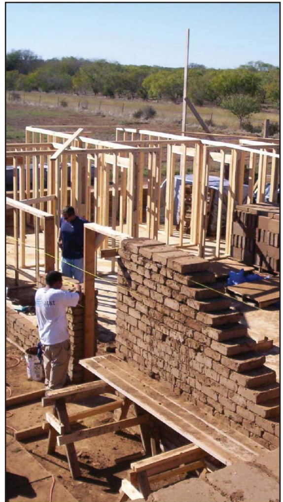
Figure 12: Hybrid construction of Compressed Earth Block (CEB) and wood stud construction. Credit: http://www.udcinc.org/CEB2.html
