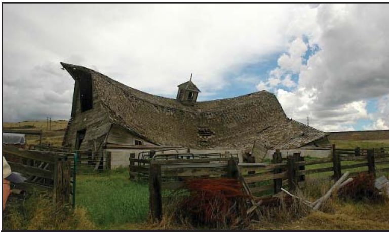
Figure 15: The Calf Creek Barn, before rehabilitation, 2009. Credit: Chris Moore, Washington Trust for Historic Preservation.
